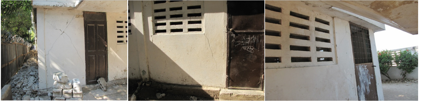
The east end of the main administration building which also houses the boys' home, the guest rooms, and the food storage depots had extensive damage. There was major damage was to the lower wall which is the supporting wall for the second floor. Taken March 2010.
